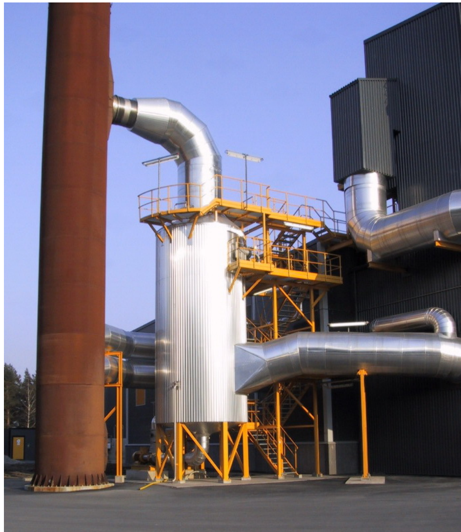
Figure – Scrubber tower, Västerbyverket, Götene.
