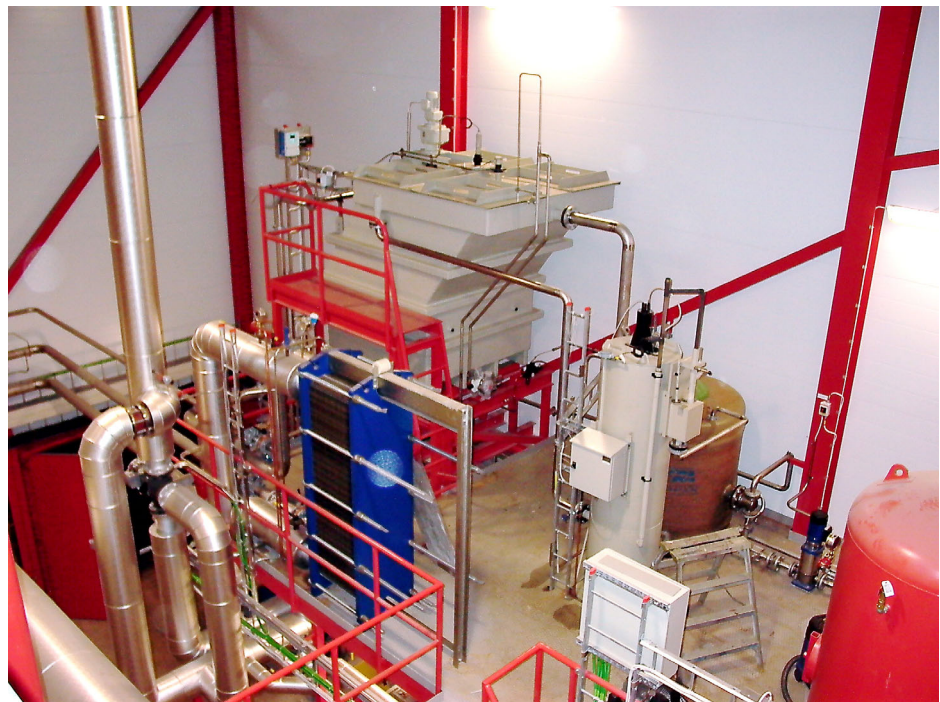
Figure – Condensate cleaning for PC Såget. Heat exchanger for district heating is also shown in the middle.
