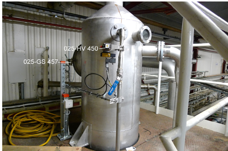
Figure – Upper part of CO 2 -scrubber for Lantmännen Reppe AB.
