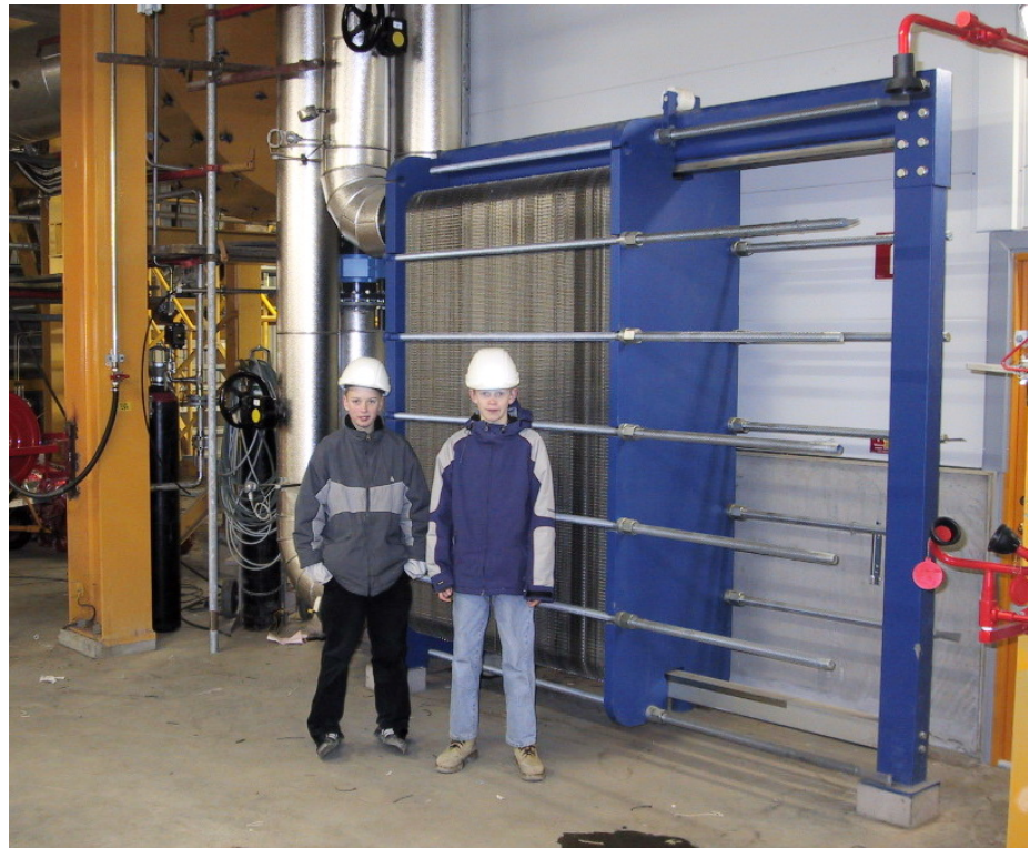
Figure – District heat exchanger for scrubber circuit. Västerbyverket, Götene.
