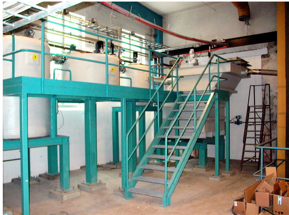
Figure – Condensate cleaning Perstorp AB.
