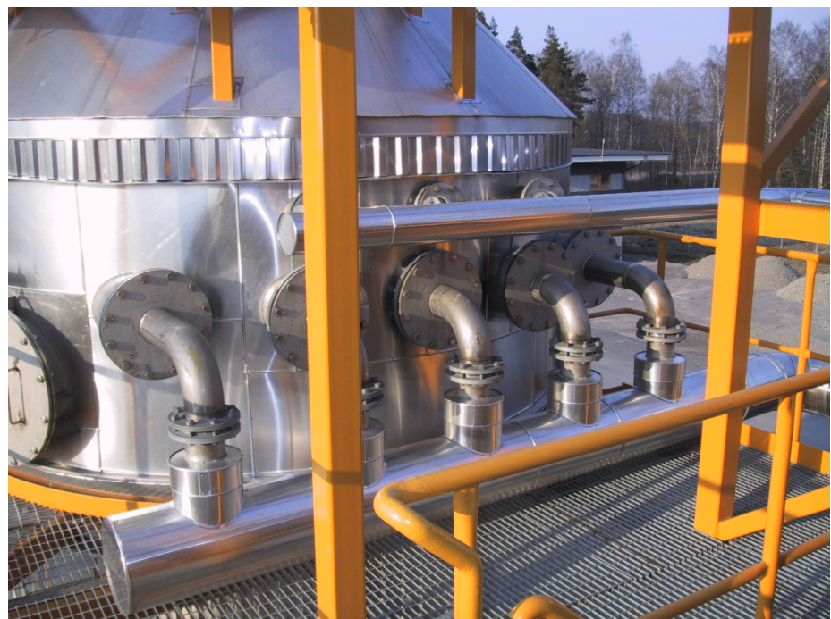
Figure – Detail, externally removable spray nozzles. Scrubber tower Västerbyverket.
