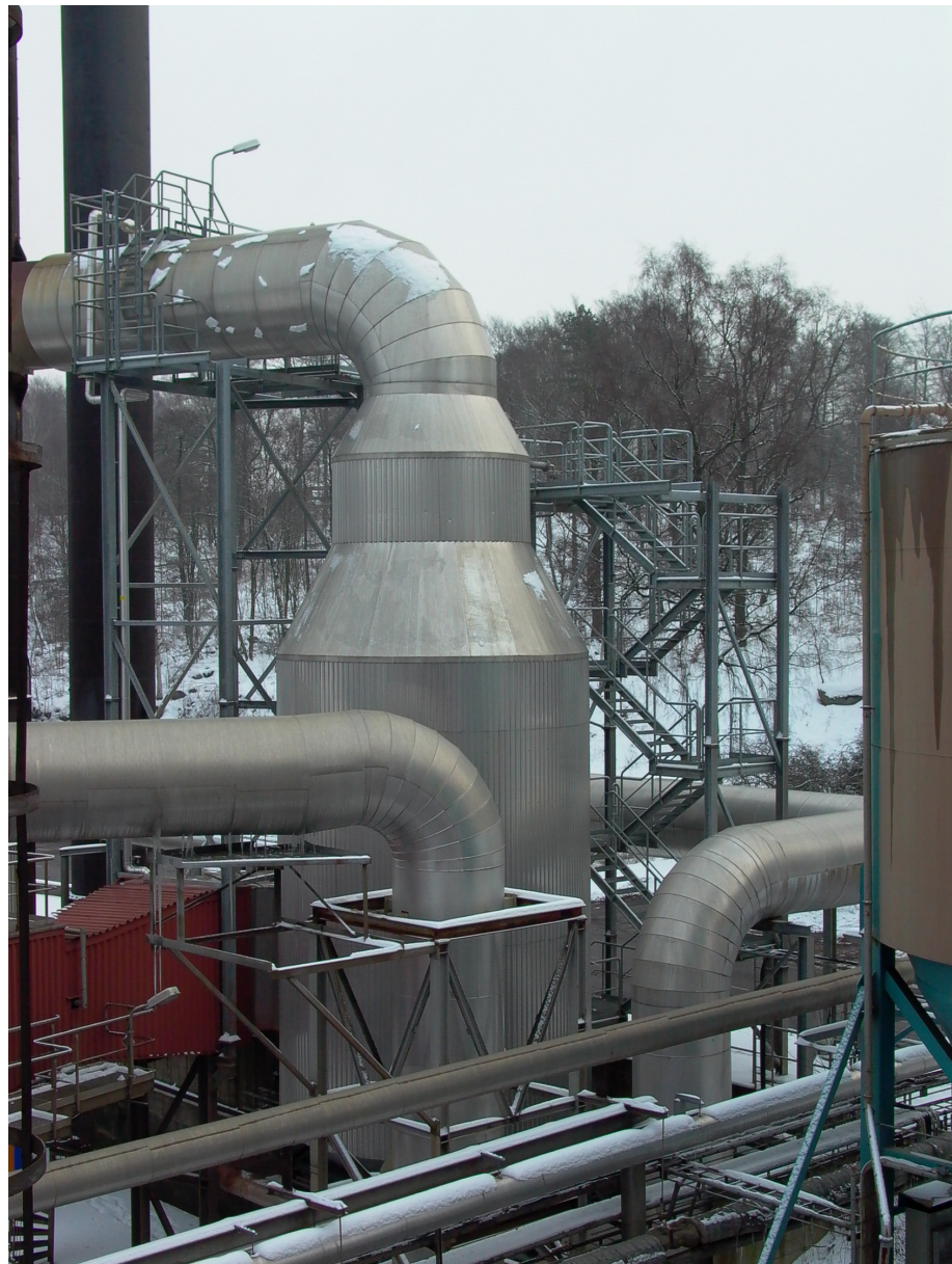
Figure – Scrubber tower at Perstorp AB
