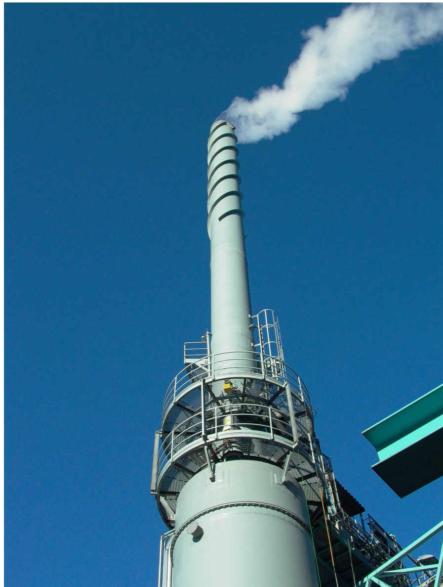
Figure – Perstorp Specialty Chemical. Combined scrubber, wet ESP, and stack.
