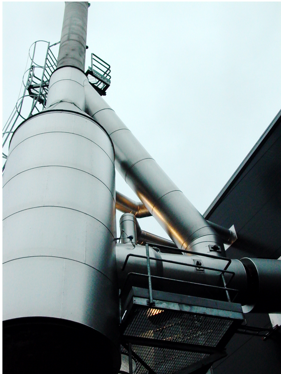
Figure – Scrubber tower with bypass. PC Såget, Herrljunga, Sweden.
