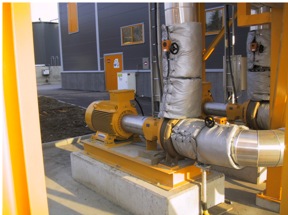
Figure – 2 x 100% capacity circulation pumps for scrubber. Västerbyverket Götene.
