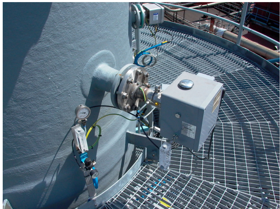
Figure – Detail of emission monitoring. Perstorp Boiler #8.
